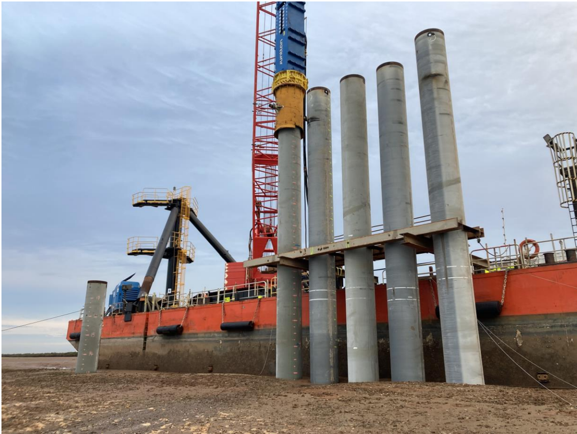
Driving the anchor piles off side of barge five at a time
