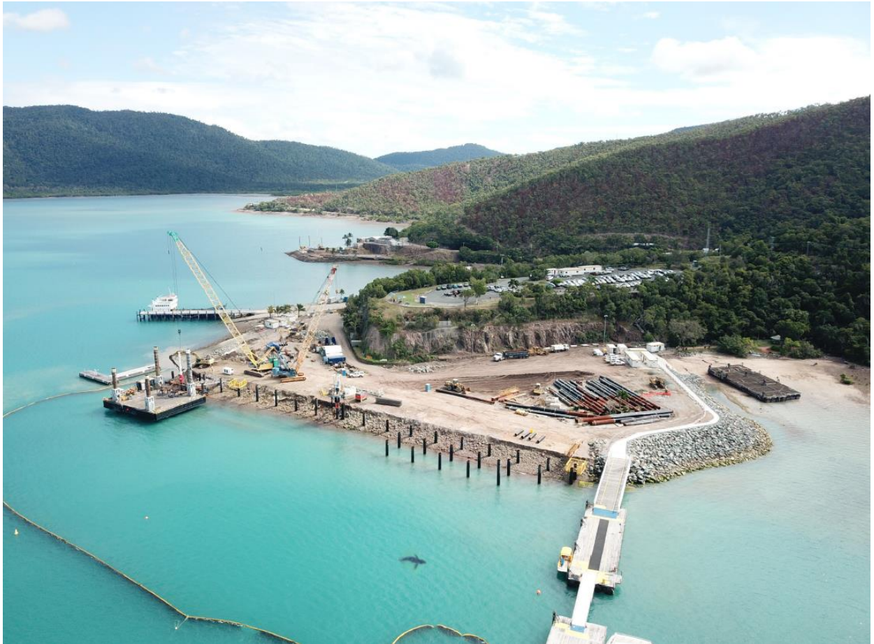
JUB and gates on left, new piles in centre and pontoons on beach far right to be repaired and reinstated
