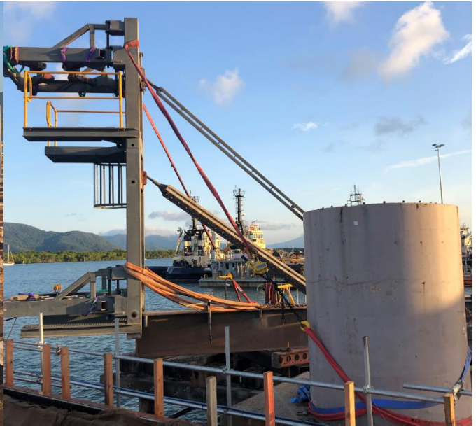
Needle beam pile gate
