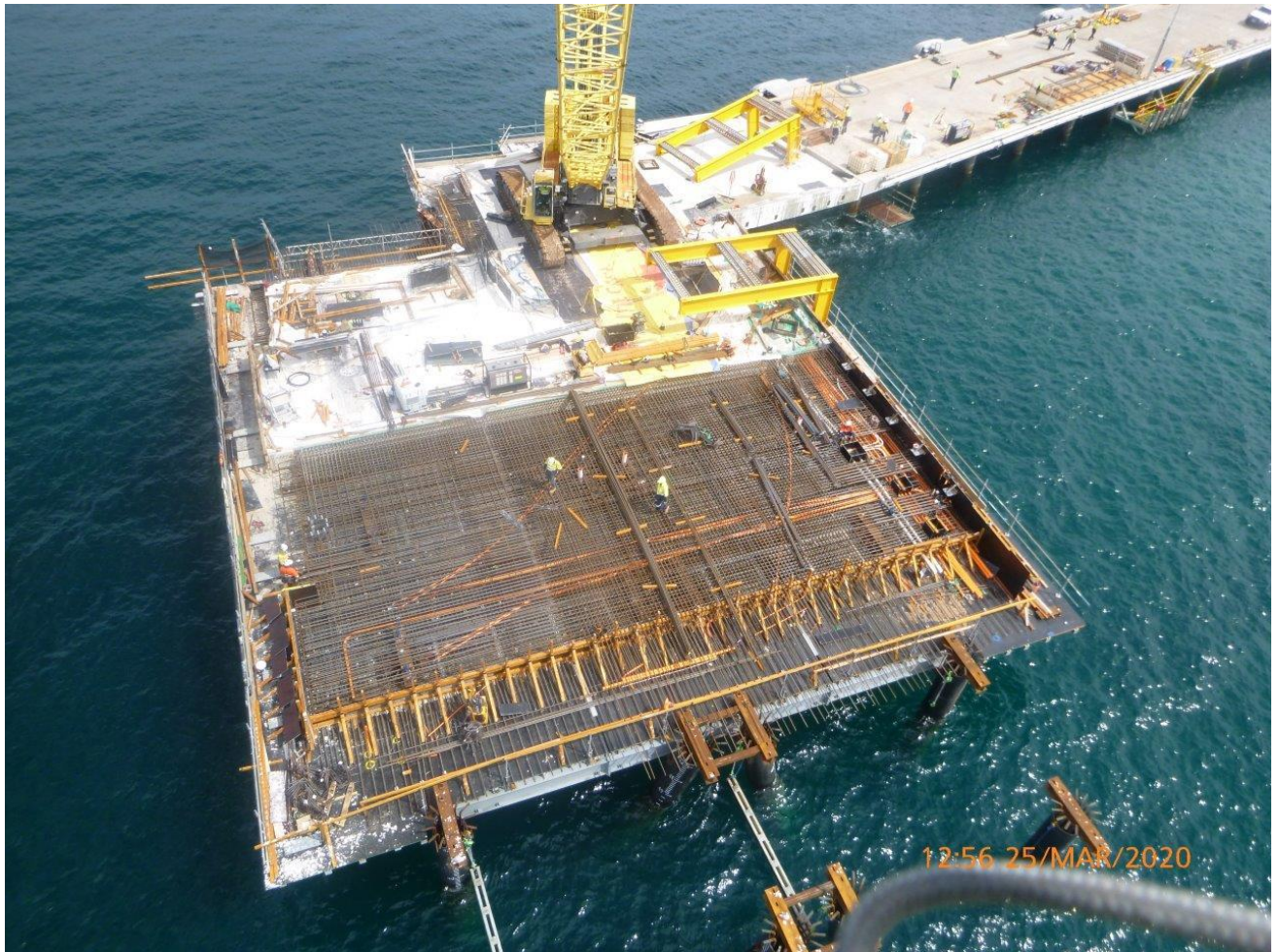
Formwork and rebar for standard 25m*12m pour, Form removal C beams next to 275t crane
