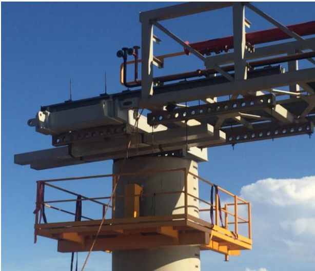
Crow's nest and Temp Support steel to place pile caps and walkways
