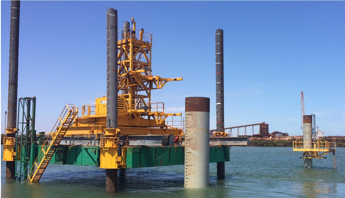
Existing pile frame mounted on jack-up barge to drive 2m diameter mono piles
