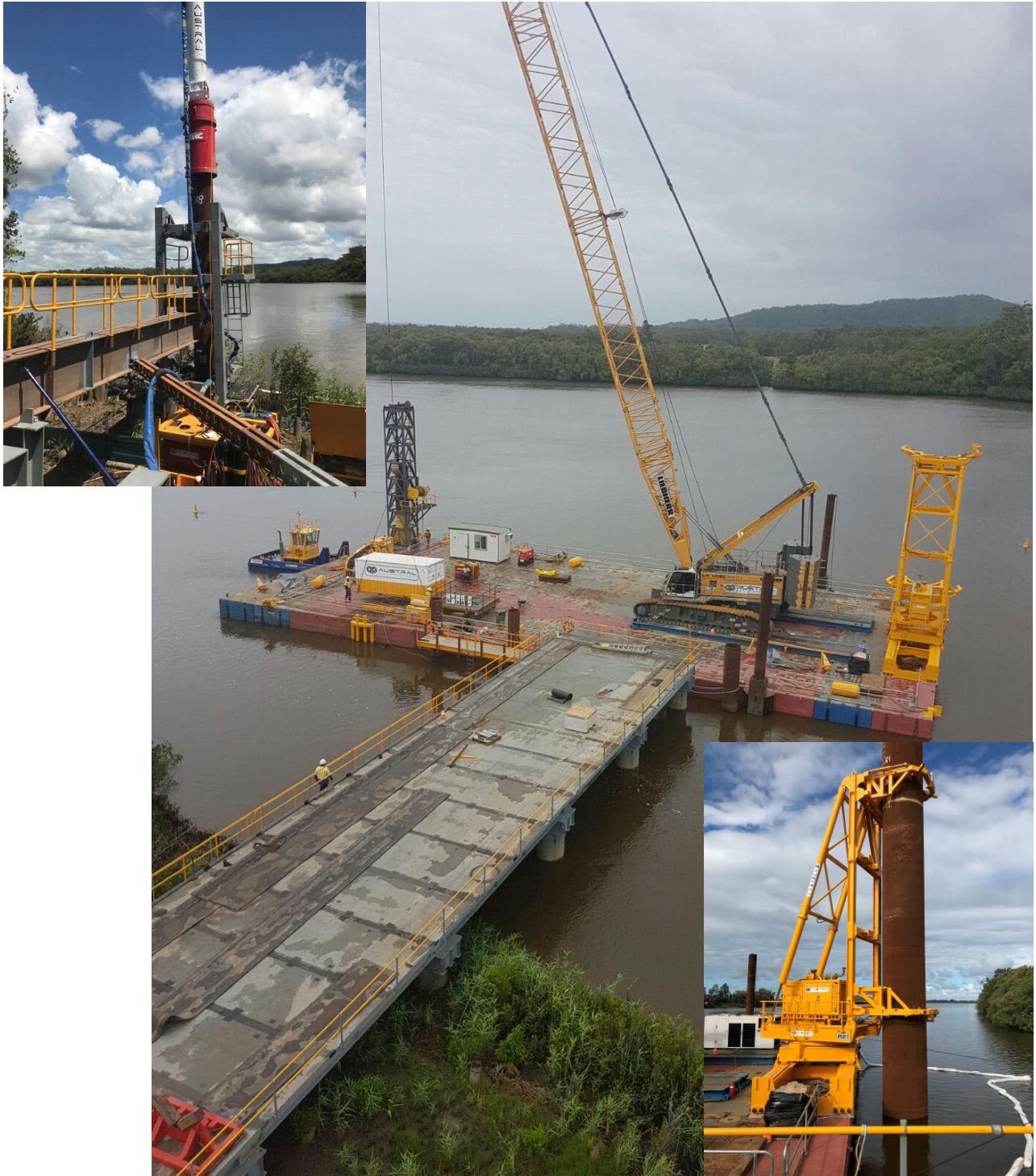
Various temporary works including piling gates, lift studies, crane mats, barge stability etc
